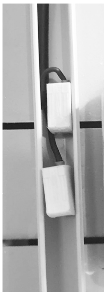
Connection in the cable duct
